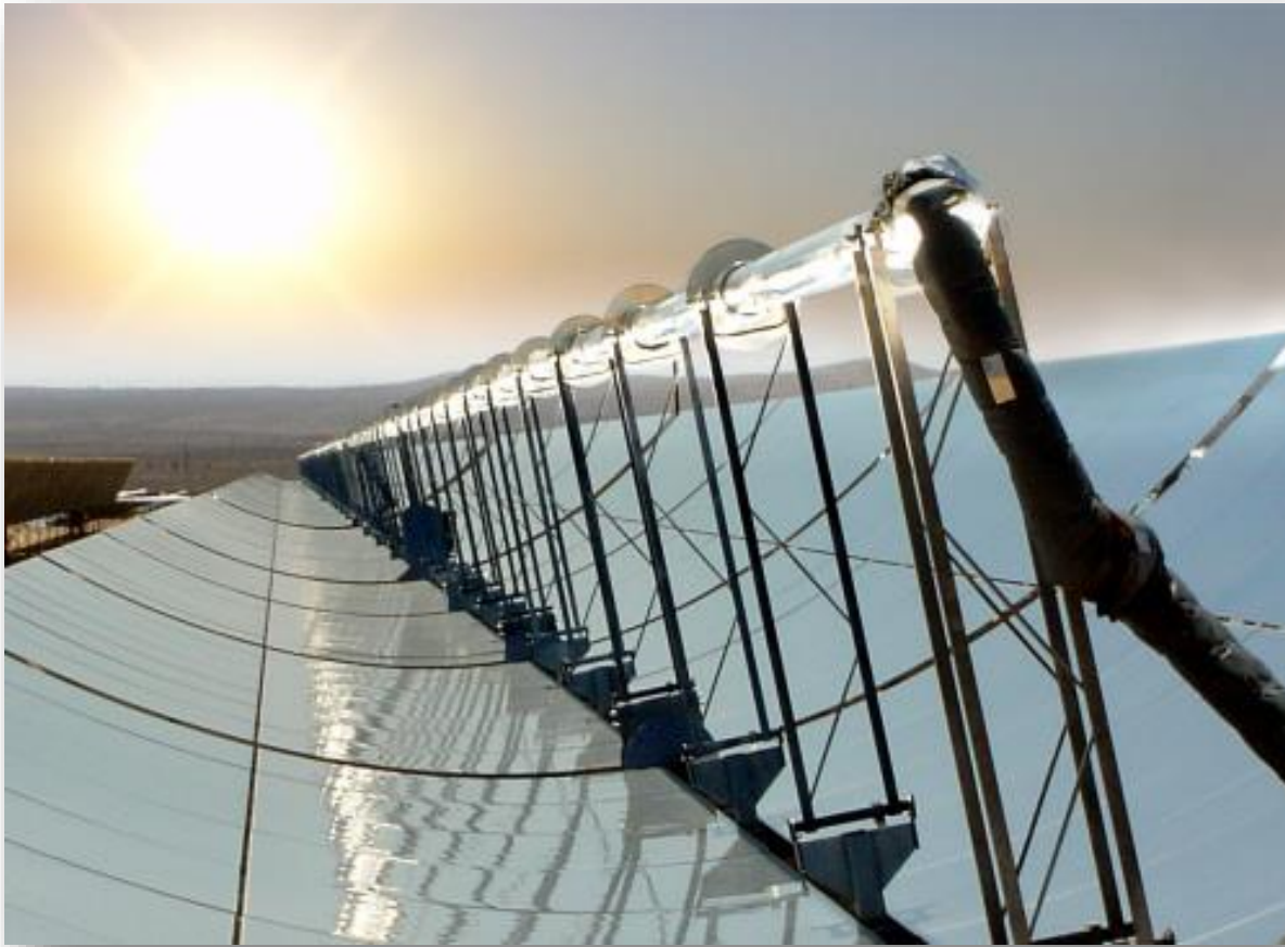
Close up view of parabolic trough and heat collector
